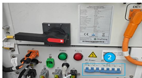
Figure 5-9: Disconnect AC/DC switches and disconnector
