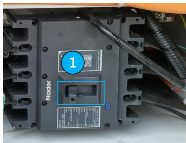
Figure 5-2: Close MCCB QF0 switch
