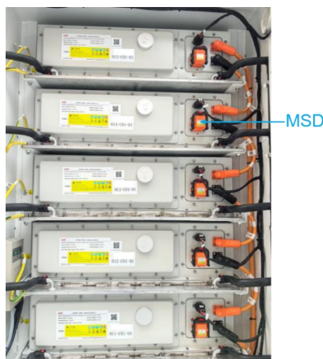
Figure 4-61: MSD installation position
