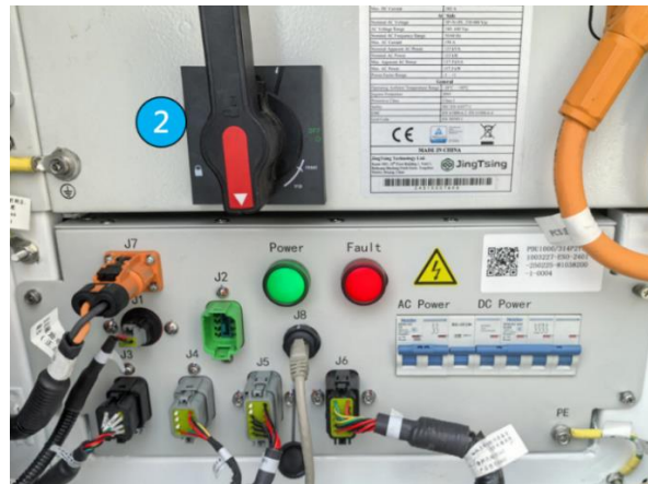
Figure 5-3: Closing PCS circuit breaker
